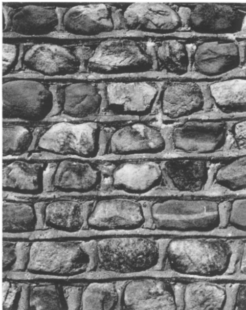
FIG. 4. Cobblestone masonry. Typical glaciated texture. (Author)
